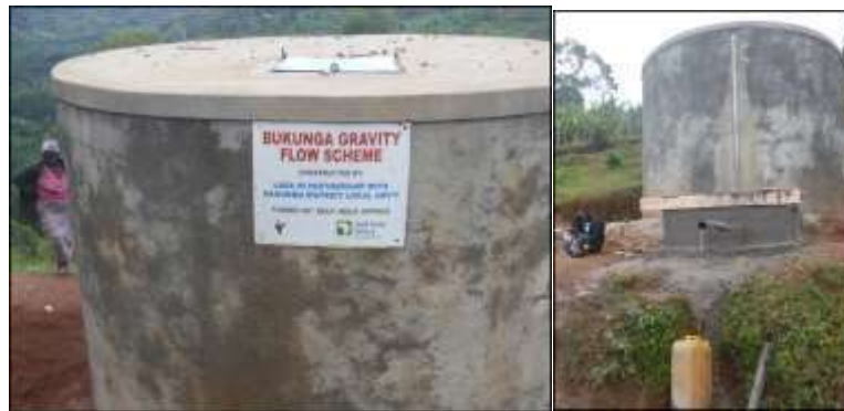
Figure 3.4: Reservoir tanks for water storage in the gravitational flow system.
