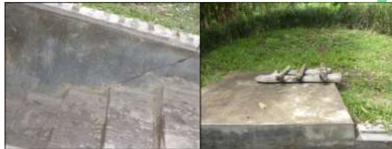
Figure 3.17: Cracked wall and the wooden cover top of the reservoir tank of one of the spring water source.
