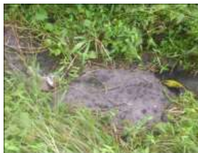
Figure 3.3: Bushy and silted drainage channel.
